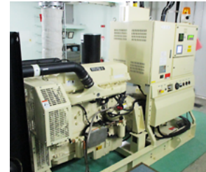
[ Emergency power generator in the telephone facility ]
